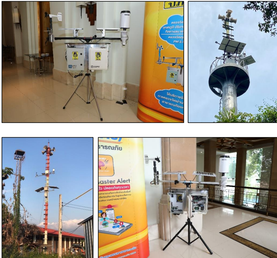
Examples of installed telemeters
